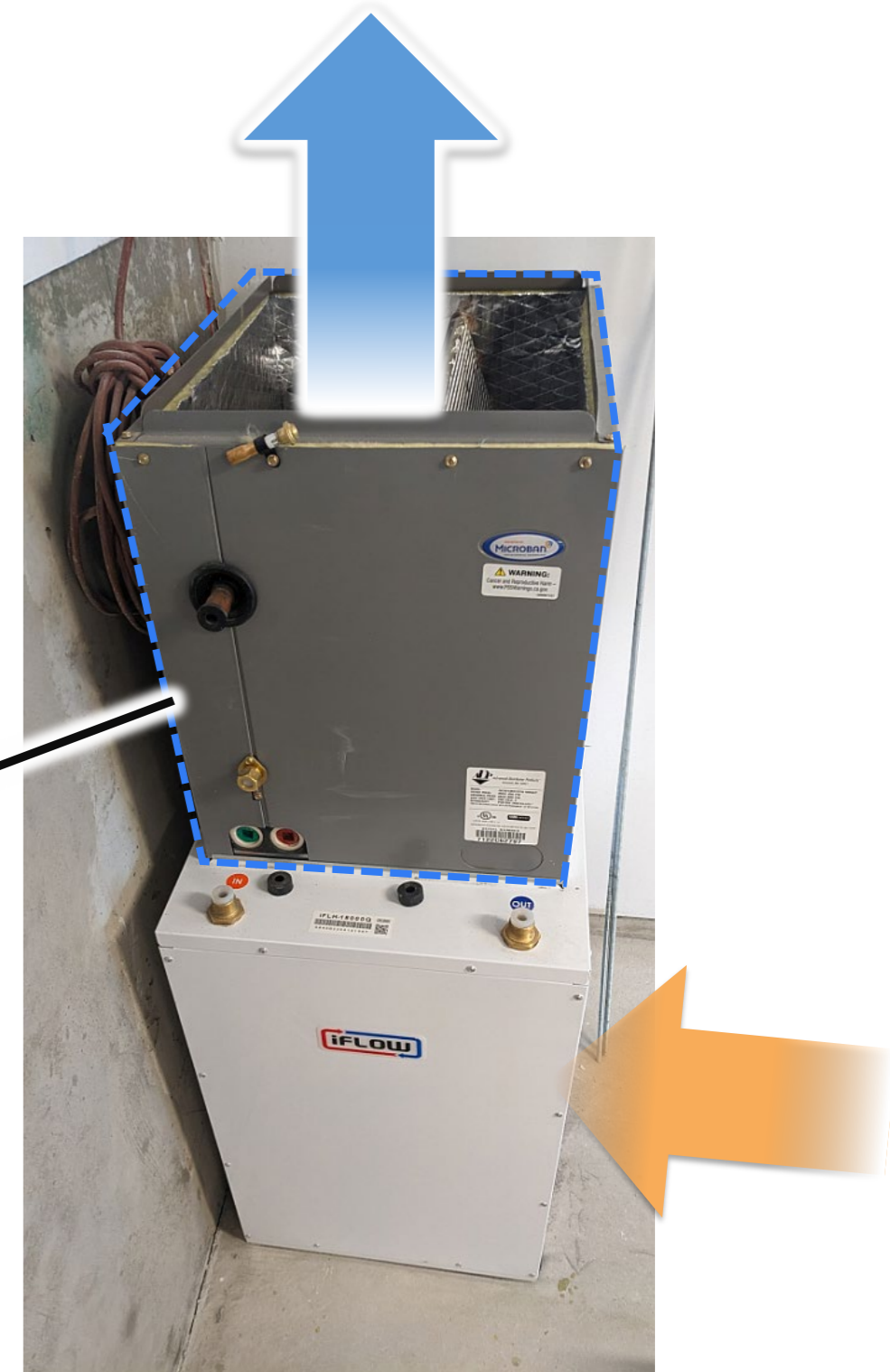
Heat Exchanger on Air Handler
