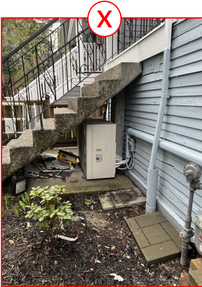
Limited clearance and restricted access for service
