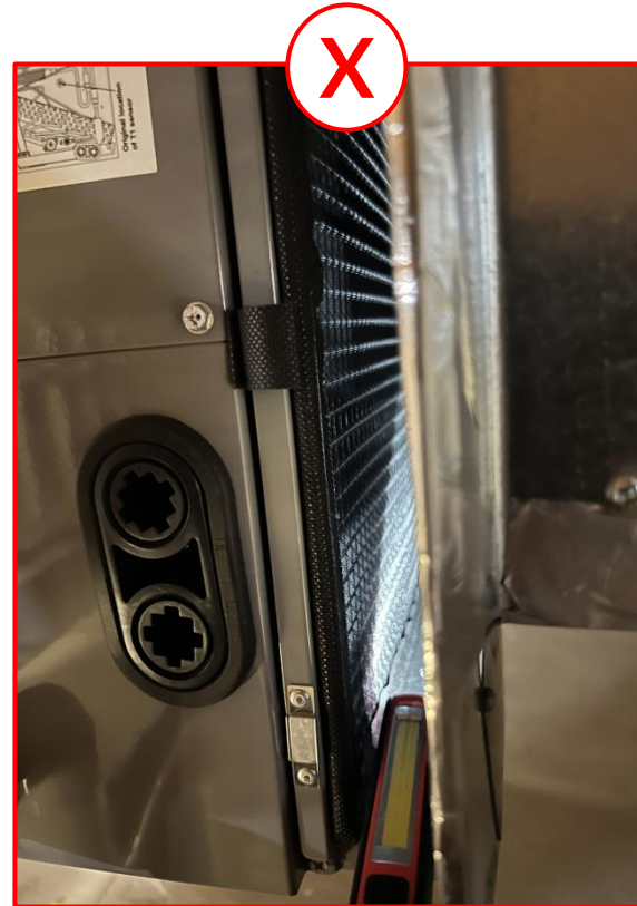
Plastic screen “filter” installed in 1” filter rack
