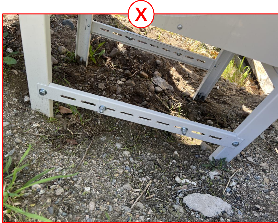
Heat pump stand on dirt with no pad and unlevel.
