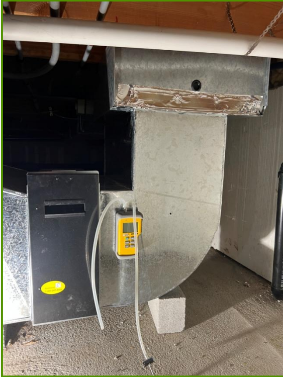
Sealed filter cabinet
